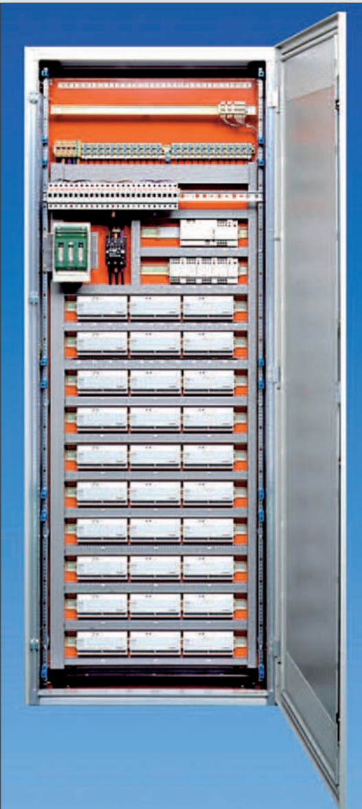
dimmer rack cabinet
